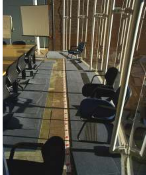
Copper tape antenna installed under carpet
